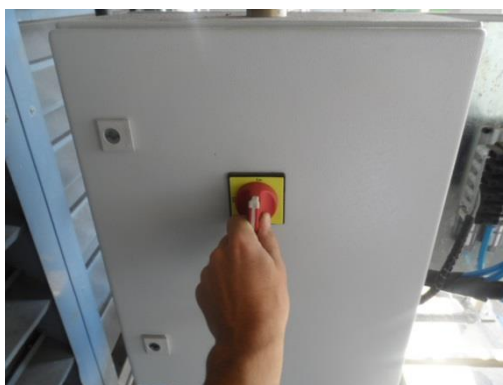
Fig. 10 – Chave geral do painel.
