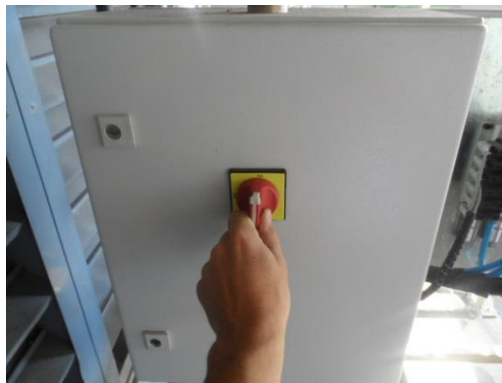
Fig. 25 – Chave geral do painel.
